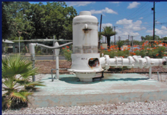
A public water supply wellhead in San Antonio, TX
