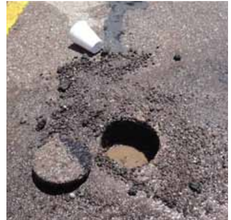
Researchers took coring samples along I-20 to determine the cause of stripping.
