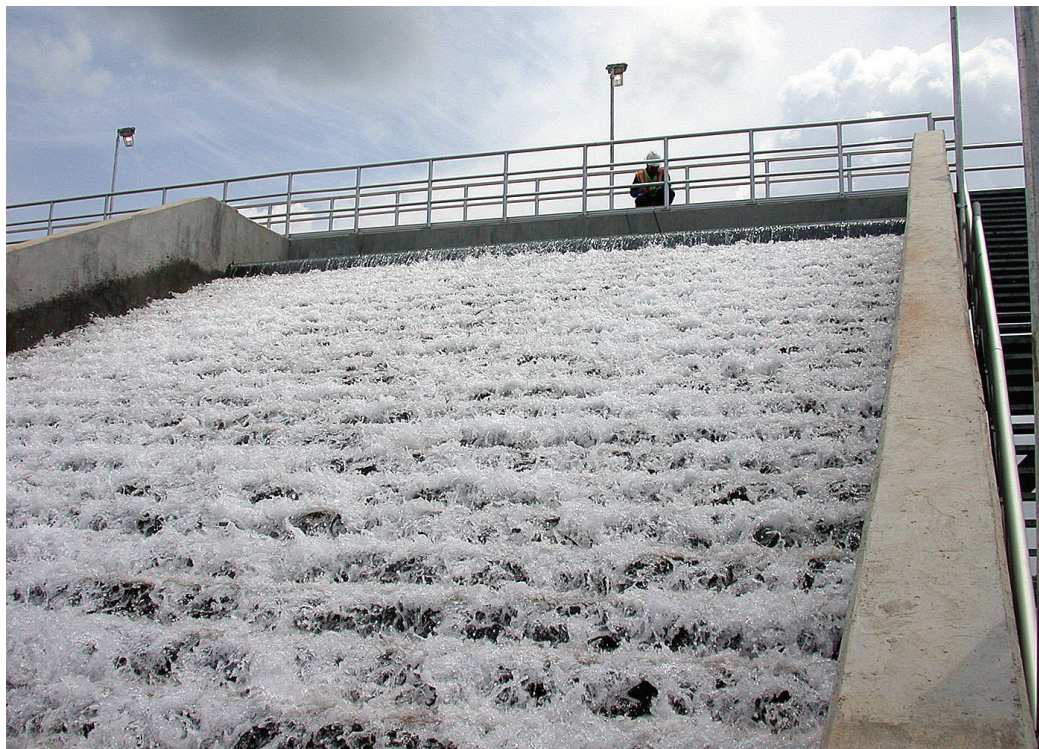
Figure 10-2. Cascade aeration, first step of treatment process.
