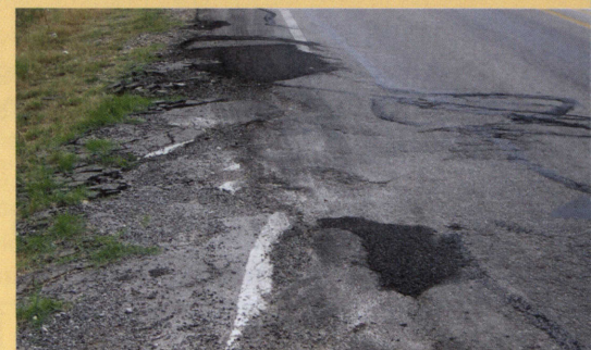
The above series of photos shows various types of pavement failures observed during field visits.
