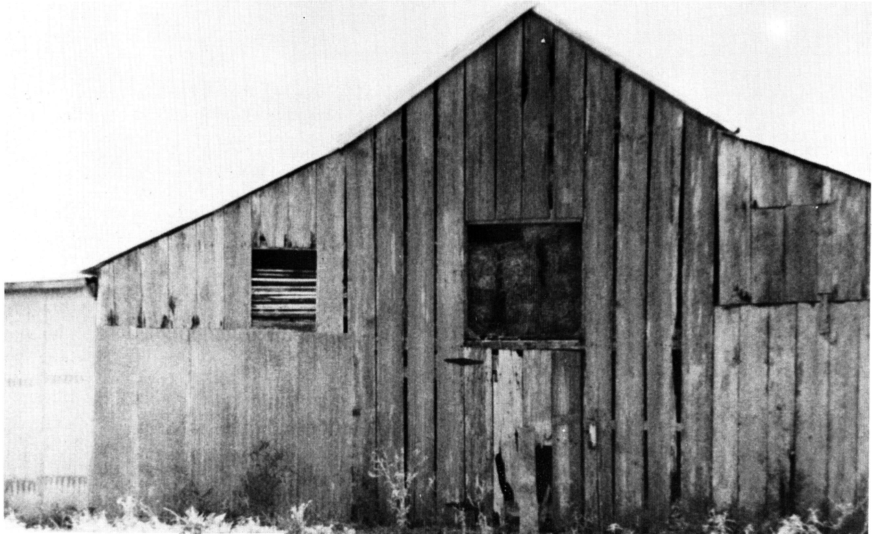
This barn was built in the early 1870's shortly after Philip and Melvina Slaughter founded their Lampasas County ranch. The barn which is still in use was built of lumber hauled from Austin by oxen.
