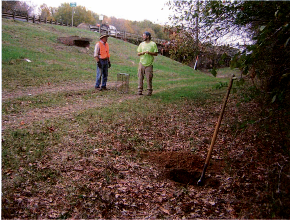
Figure 12 Shovel Test 32 looking east at left bank abutment of the Sabine River bridge on SH 322/149. There will be a bore pit here for crossing under the Sabine River.
