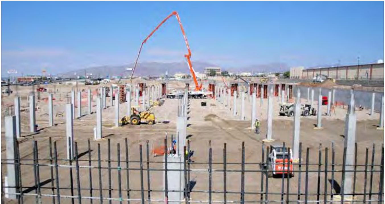
Construction of the “The Fountains at Farah” project in El Paso PHOTO: Courtesy of Centergy Retail, LLC.
