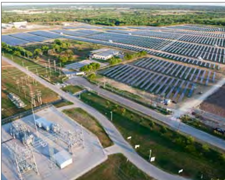
A new solar energy complex south of San Antonio produces enough power for about 2,550 averaged-sized houses a year.
