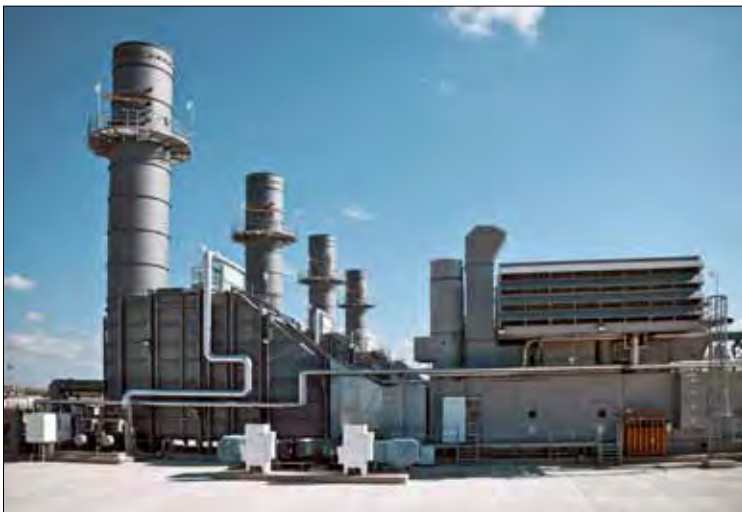
CPS Energy's Braunig Power Station southeast of San Antonio. PHOTO: Courtesy of CPS Energy and the San Antonio Economic Development Foundation
