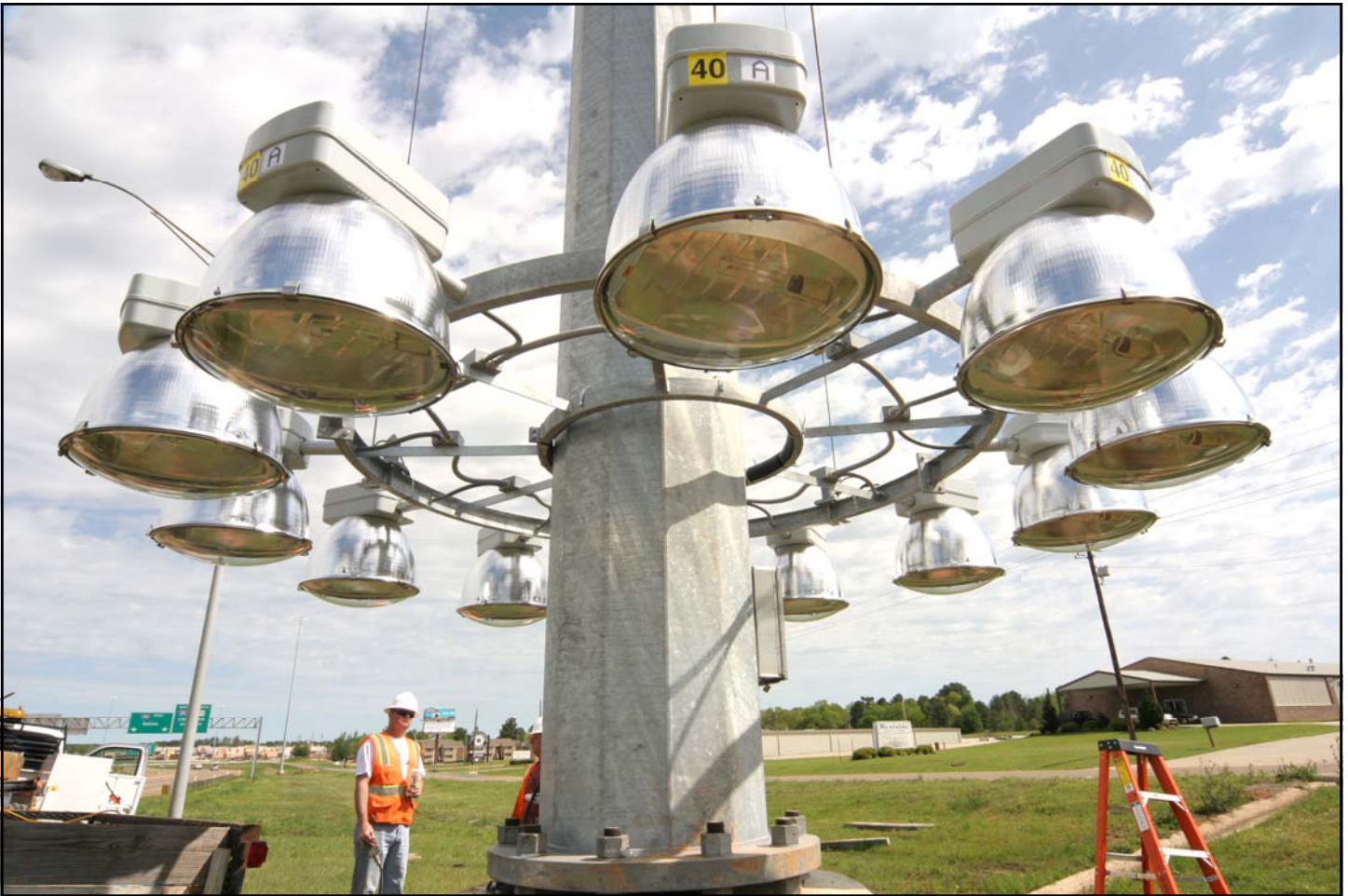
Workers prepare to raise the high-intensity lighting fixtures on a high mast near Loop 151. The lighting fixtures are made where they can be lowered for easier maintenance.
