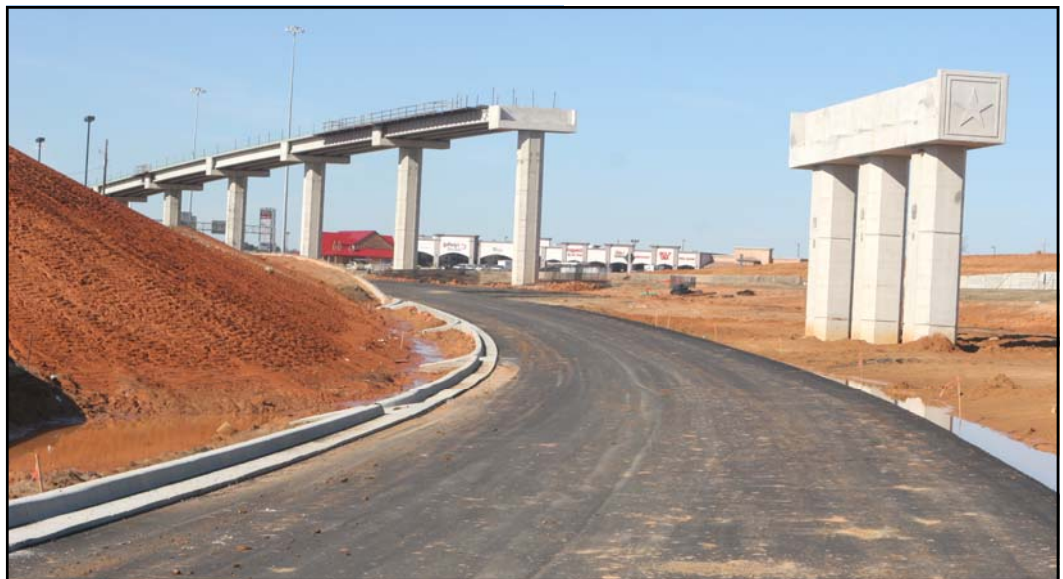
Base materials are finally down on the new section of frontage road between New Boston Road and Pecan Street on the south side of Interstate 30 and crews continue to construct the bridges and overpasses that will be part of the big interchange at Loop 151.
