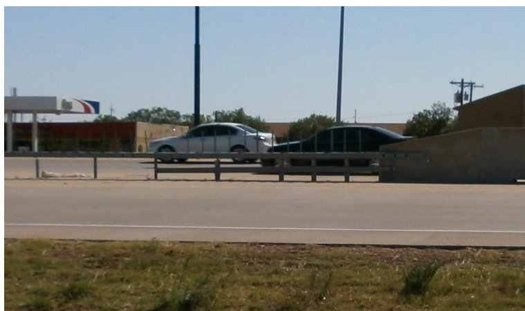
Figure 4.3. A Steel Beam with Support Posts Is Used instead of a Concrete Barrier for the Portion of the Divided Highway That Is within the 100-Year Floodplain.
