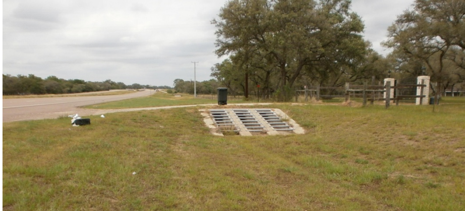
Figure 4.9. Mounding above Driveway Pipes Contributes to Flooding of Roadway and/or Private Property.
