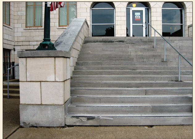
Above: Structural deficiencies at the Hunt County Courthouse in Greenville; Below: the restored 1901 Harrison County Courthouse.
