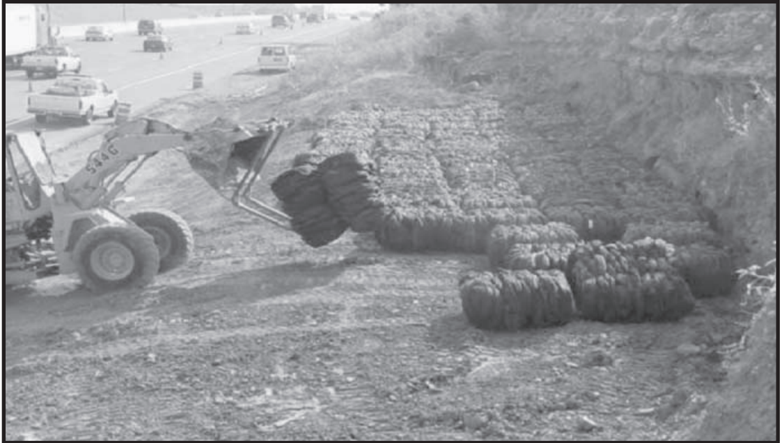
A layer of bundled recycled tires is stacked along I-30 prior to adding a layer of soil to repair an eroded slope.
