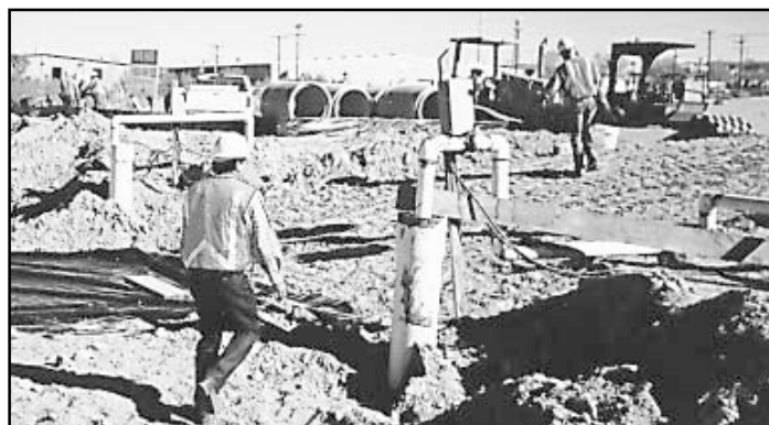
El Paso District Photo Dewatering to lower water table for storm sewer installation
