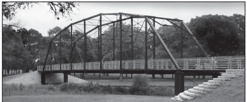
Oak Forest Bridge relocated to Kerr Creek in the City of Gonzales.
