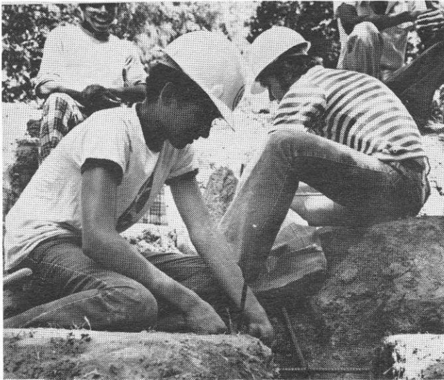
Laying the groundwork for an amphitheatre in Starke Park, these YCC participants are part of the Seguin Project.
