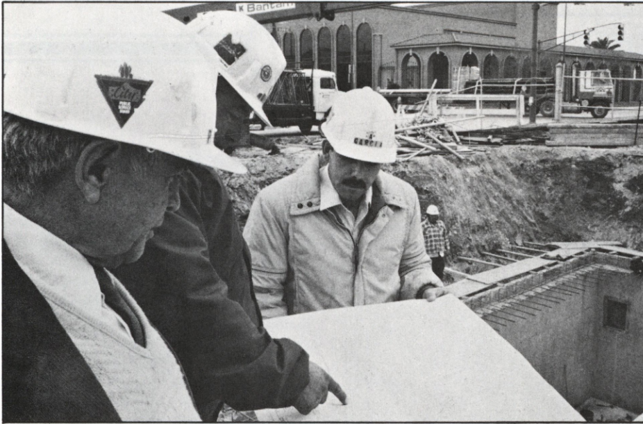
Construction Foreman Armando Montez (center) clarifies questions on vault drawings with Garcia (right) and Traut.
