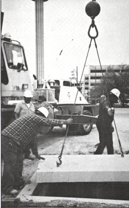
Hinojosa (left) and Wright (right) help lift lid off Marriott vault, so transformers can be installed.
