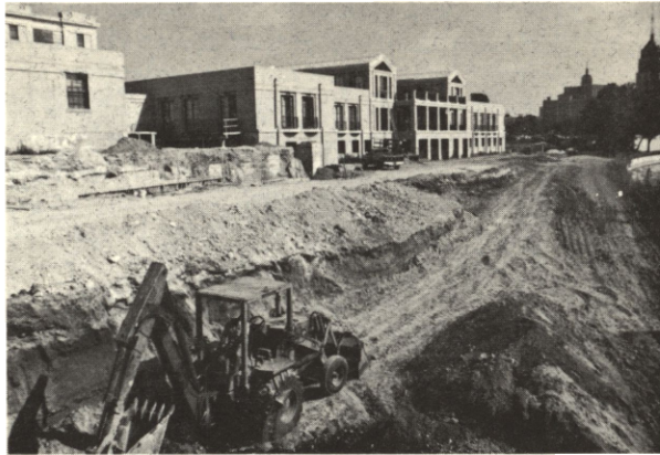
Channel Improvements Project — Betterments II presently under construction in front of the new H.E.B. Corporate Headquarters.
