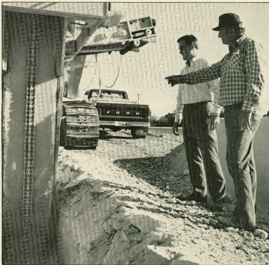
Mike Kotara , Engineer and Chief Planner of North Gate Pipeline Project, (left) and Ferdinand Kotzur , Main Crew Foreman and construction inspector, watch a rock trencher break through rocky ground in northern Bexar County.
