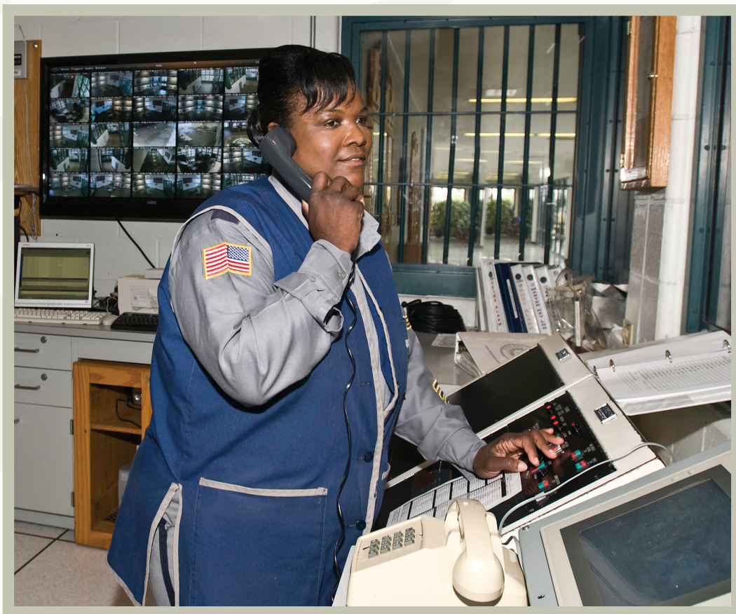
CO V Emma Williams monitors surveillance cameras on a large video board inside the control picket at the Polunsky Unit in Livingston.
