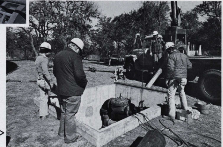
Workers are installing replenishment valves at the Bitters Pump Station. These valves will allow the tank to be filled by remote control.
