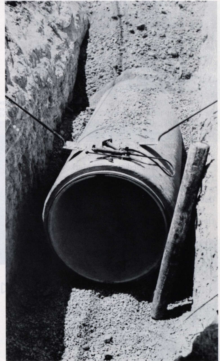
A section of 60" water main pipe. The shovels give an idea of the size of the trench and the pipe.
