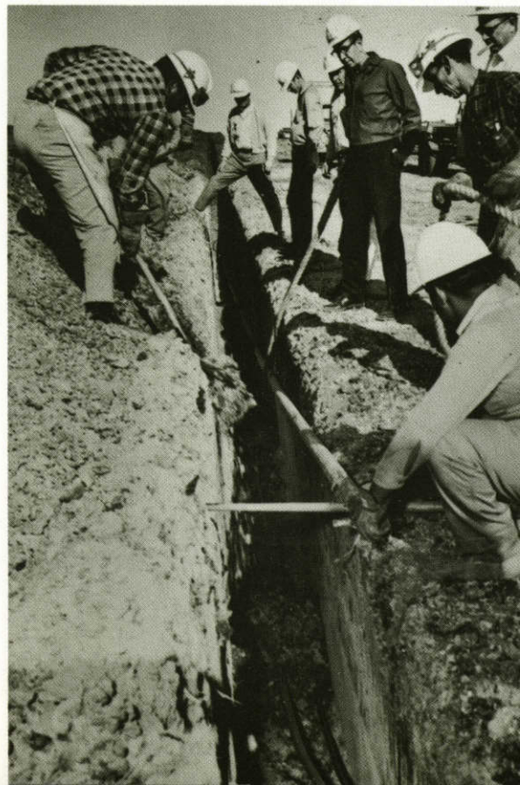
Joint trenching for gas and underground electric service is economical in rocky areas.
