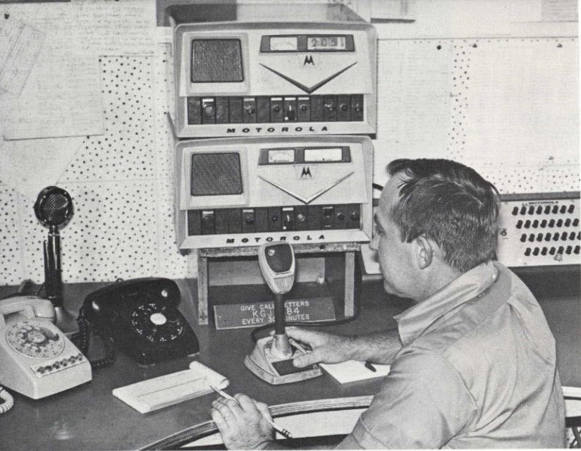
(Left) The radio dispatcher's area is the busy nerve center through which orders and information are dispensed to and received from crews manning the City Water Board's fleet of 128 radio equipped vehicles. This constant radio contact with all field units provides for efficiency, mobility and great savings in time to the daily benefit of the community.
