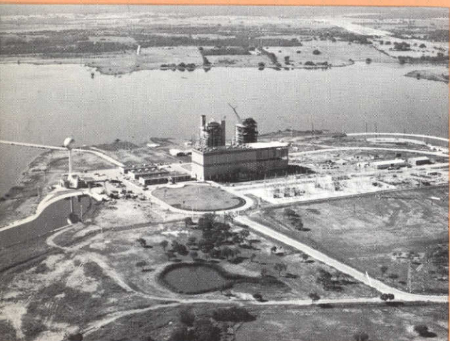
Aerial view shows first unit completed and second under construction. It will be completed in May, 1968.
