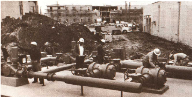
▲ Natural gas for HemisFair's chilled water plant is served from this installation.
