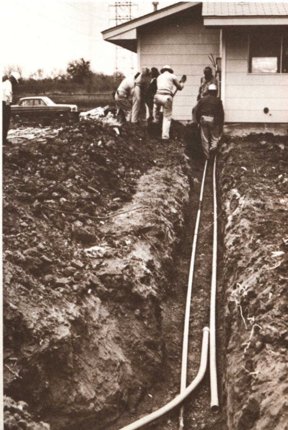
▼ Joint trenching of gas and electric service takes place in URD project.
