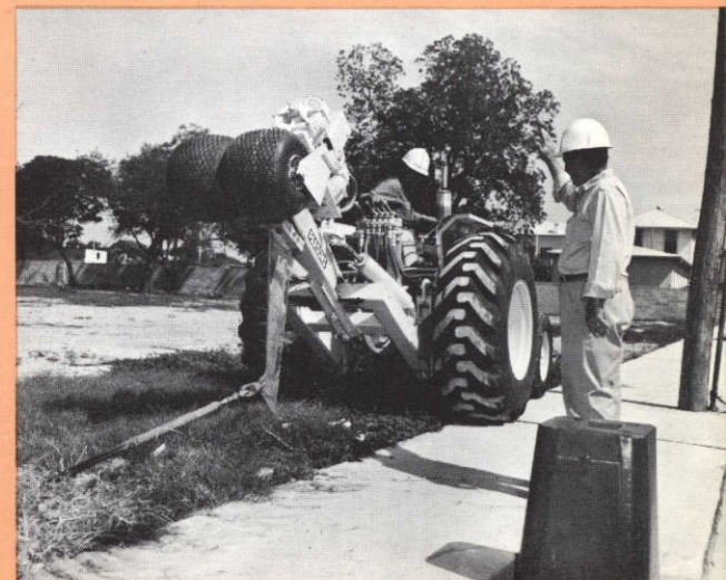
Two hydraulically operated plows like this speed URD work and cut costs.
