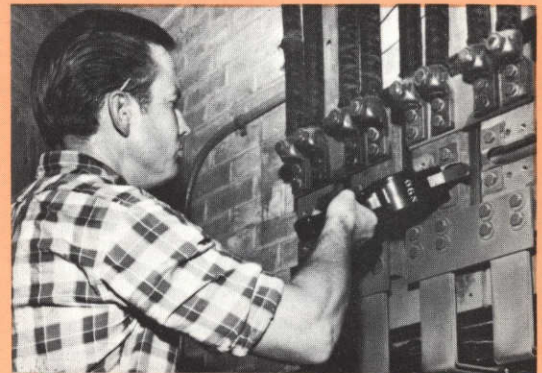
Amperage readings being taken at a downtown building.
