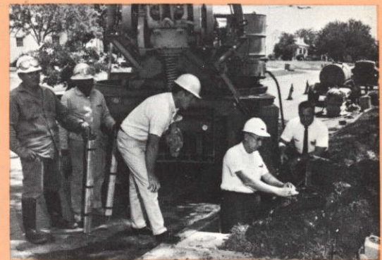
Constant vigilance: cathodic protection for San Antonio's gas mains insures corrosion free mains.
