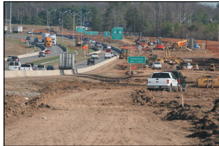
Construction work has begun on clearing the rights of way to fill in the frontage road gaps. This section of work is being conducted between FM 989 (Kings Highway) and US 59.
