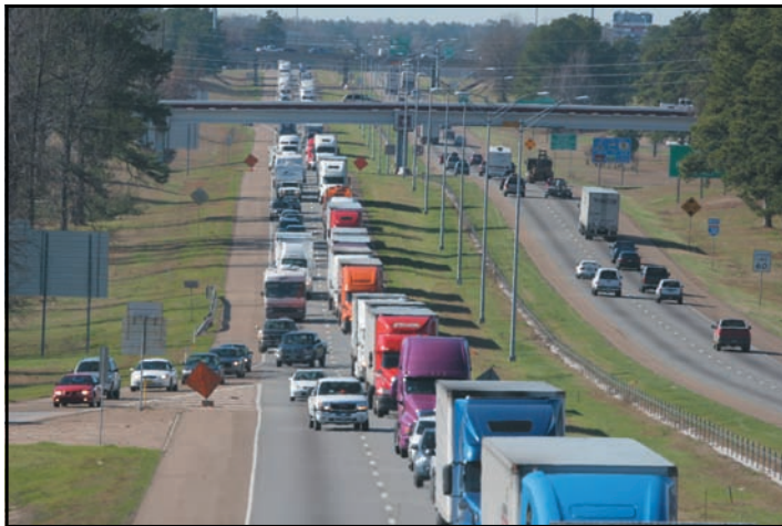
Traffic on Interstate 30 also suffered from periods of congestion as workers installed protective concrete barriers along the highway where they will be working close to traffic.
