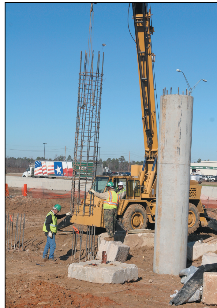
Workers prepare a rebar support for columns that will be part of the bridge crossing Interstate 30 at University Avenue near the new Gander Mountain store.
