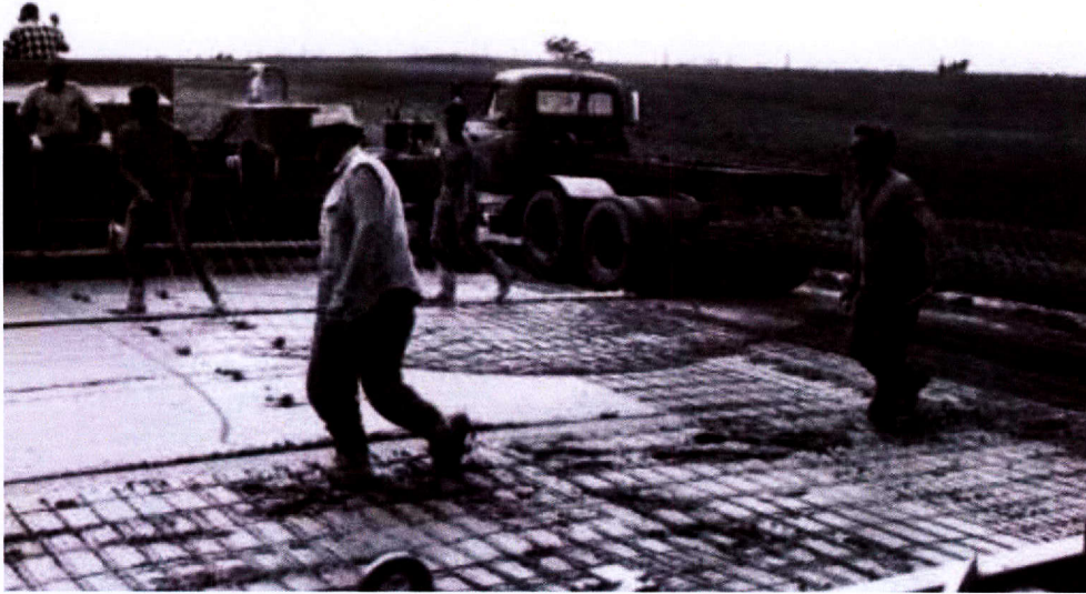
Figure 3. 2LCP with Welded Wire Mesh Reinforcement (I-80 Dallas County, Iowa 1966) (Grove and Taylor 2010).
