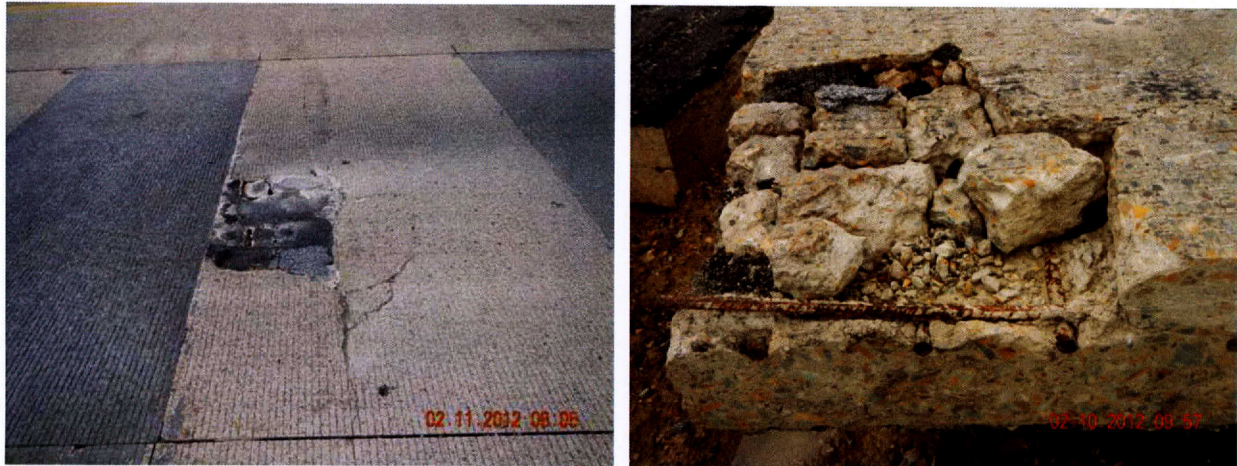
Figure 8. Two-Lift Pavement Delamination on I-30 at Sulphur Springs, TX (Photo Adopted from Dr. Moon Won).
