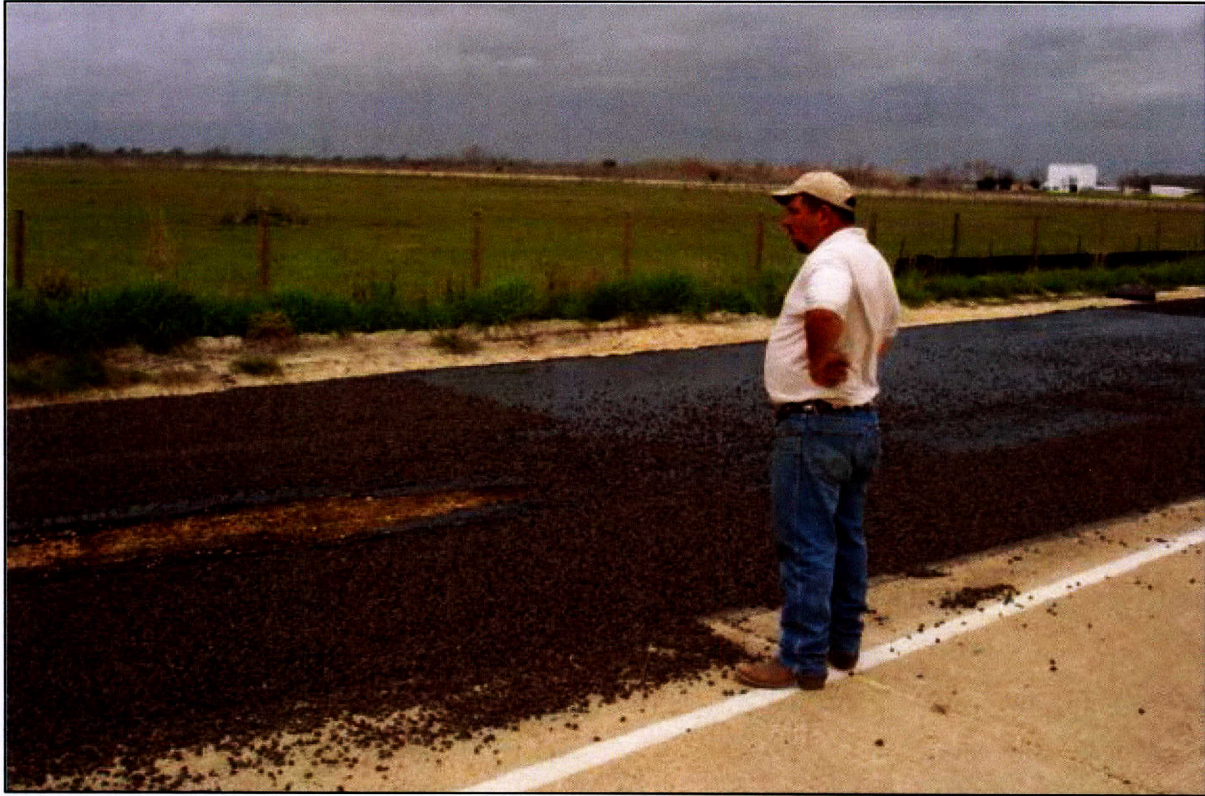
Figure 48. Strip of Grade 3 Course that Peeled Off at South Access Ramp.
