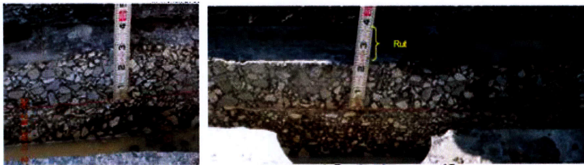
Figure 1-1. Forensic Evaluations on US 79 (Bryan District) due to Premature SMA Rutting (about 1.2 inches Surface Rutting).
