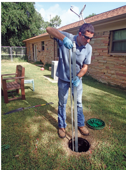
Inspection of an On-Site Sewage Facility - Courtesy of Texas A&M Agrilife Research
