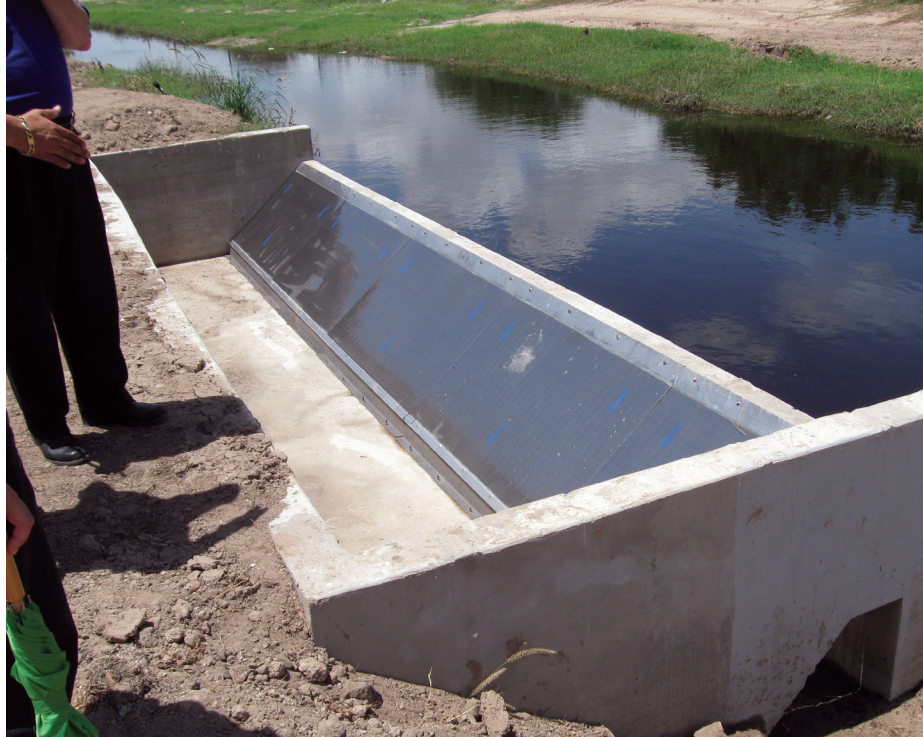
Microscreen filter installed upstream of a stormwater detention facility in McAllen.
