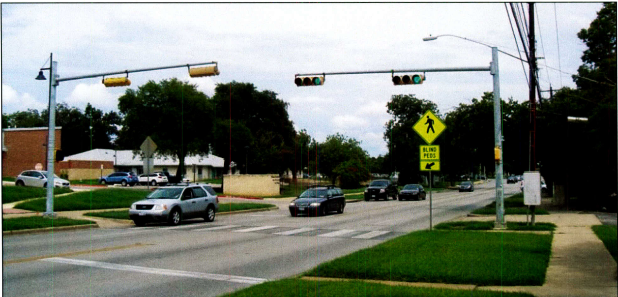
Figure 6. Example of Traffic Control Signal Installation.
