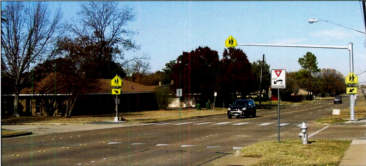
Figure 9. Example of Rectangular Rapid-Flashing Beacon with School Crossing Sign Installation.
