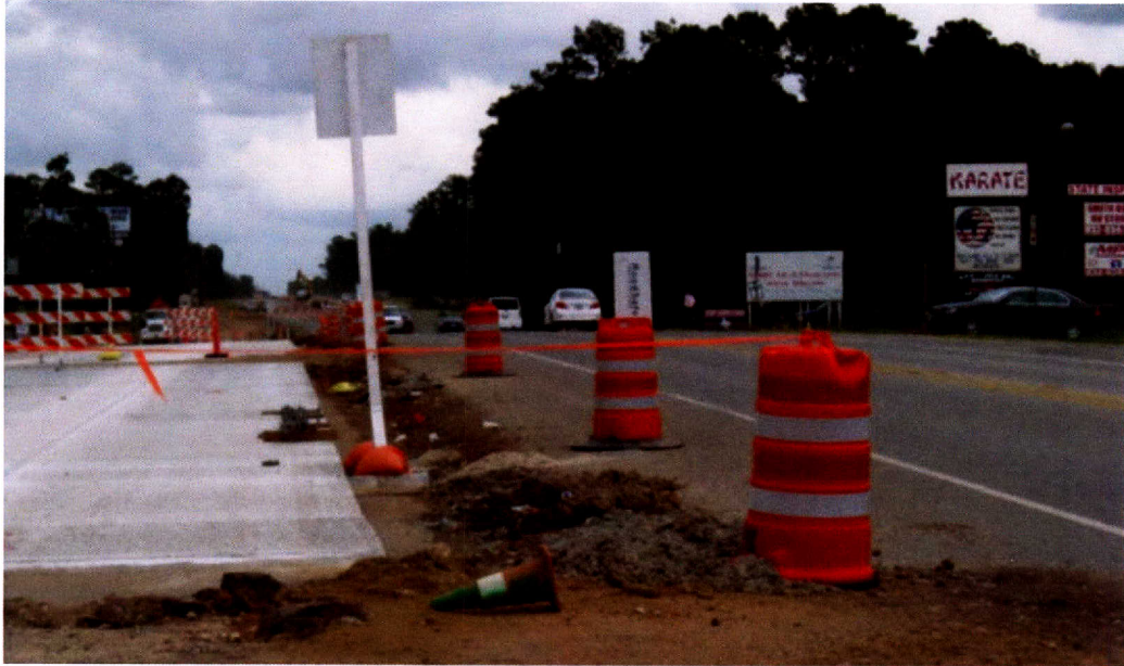
Figure 2. Driver's View from a Passenger Car in a Driveway in a Texas Work Zone (3).
