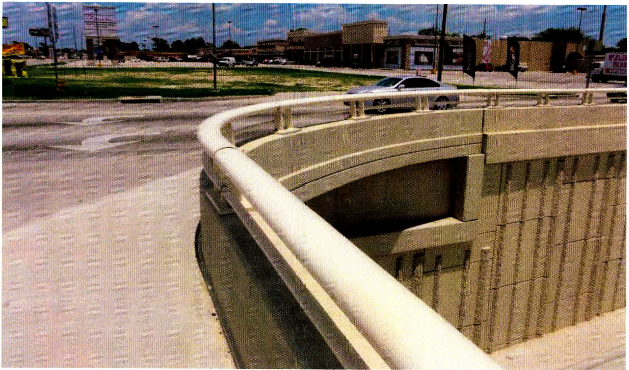
Figure 3.29: View of nearest location for moisture infiltration, at southeast corner of intersection.
