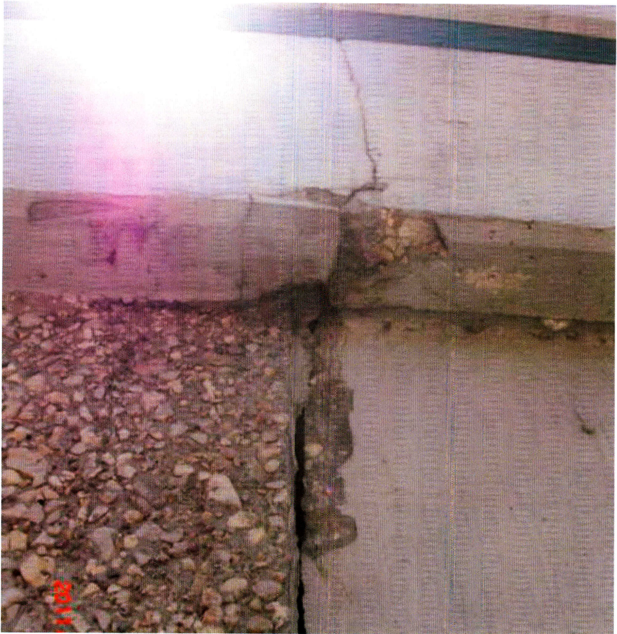
Figure 3.38: Some cracking was seen at the connection between two facing panels on the southwestern portion of the wall.
