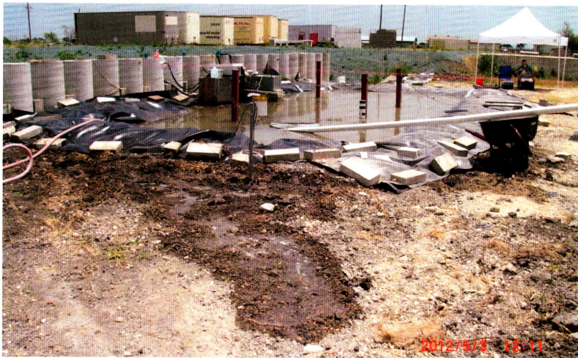
Figure 4.37: Leakage from west side of inundation zone.
