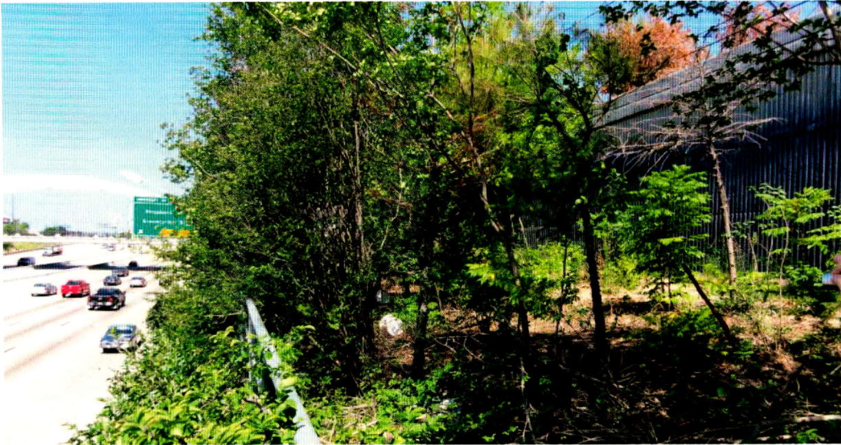
Figure 3.33: Approximately 40 feet of exposed soil behind the wall near Hazard Street (facing west).
