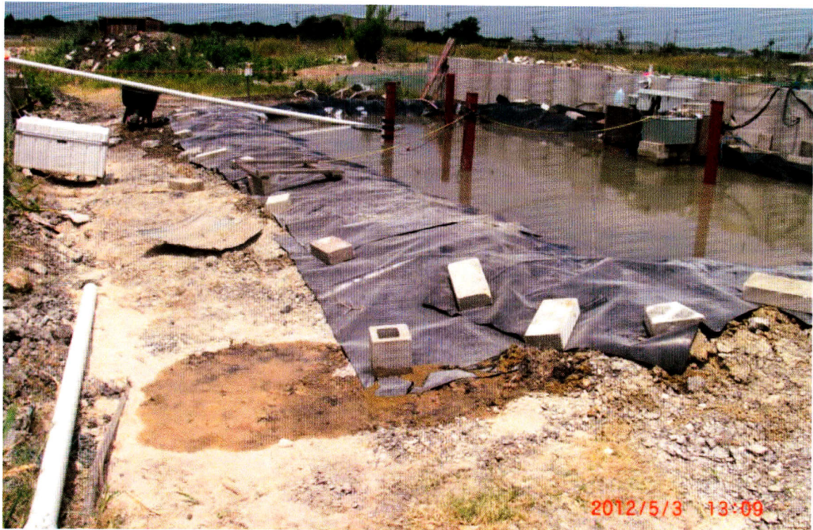
Figure 4.36: Leakage from southeast corner of inundation zone.
