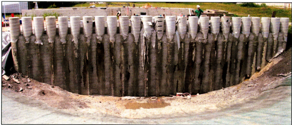
Figure 5.38: Water infiltration into the excavation was first observed 90 minutes from the start of inundation.
