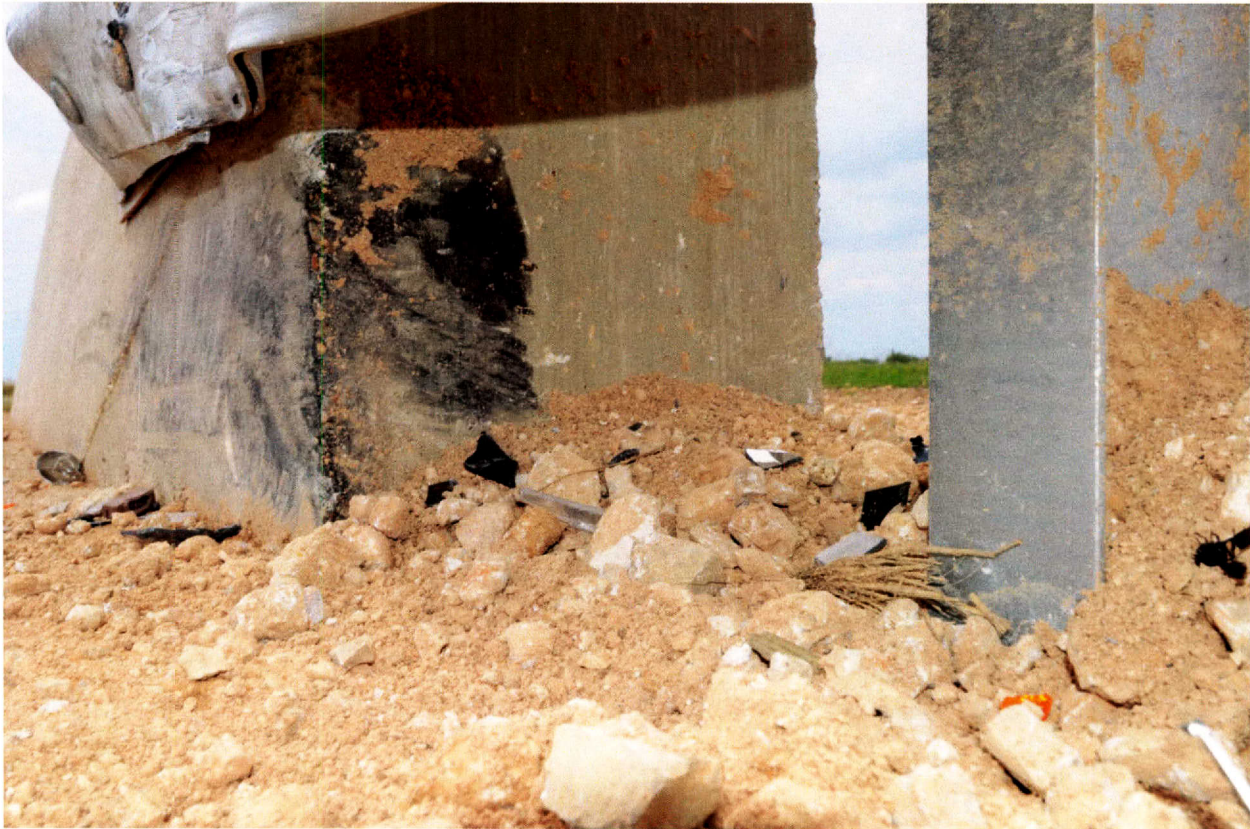
Figure 5.3. TxDOT TL-3 Transition after Test No. 490022-4.
