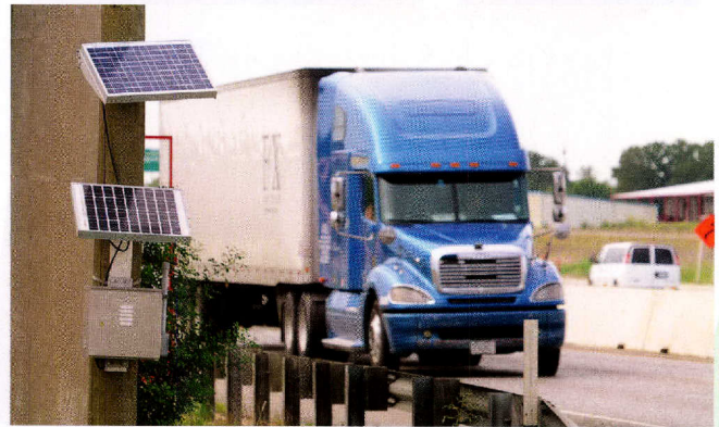
TTI’s AWAM technology is installed inside a box on a utility pole near Hillsboro on I-35, helping agencies measure travel times and improve mobility.
