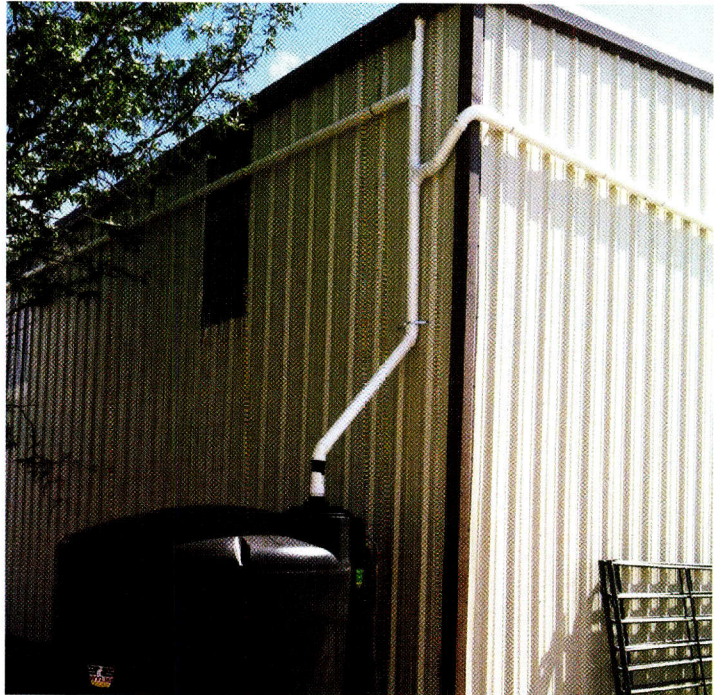
PGCD's newest rainwater harvesting addition on the shop.
