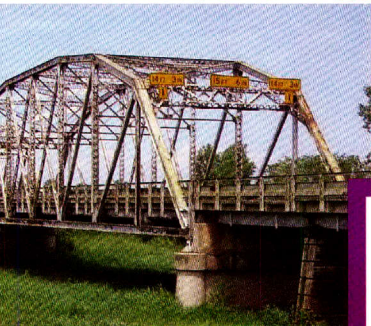
The Salt Fork of the Red River Bridge before it was demolished.
