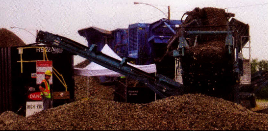
NorthGate Constructors breaks down concrete and recycles it for use as a base with new pavement. Since this process occurs on site, it saves time, requires fewer trucks and diverts less material to landfills.
