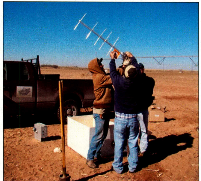
David Martinez, of the Texas Water Development Board, assists PGCD personnel with the installation of a satellite monitoring well.
