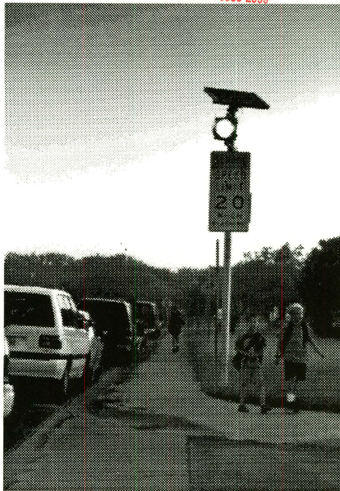
School crossing signal powered reliably by PV Photovoltaics are a perfect solution for situations calling for small amounts of power and high reliability.
