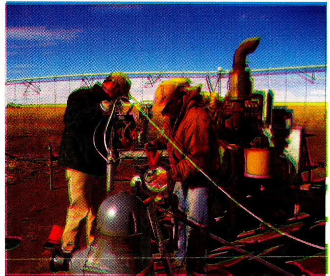
Field Technicians Devin Sinclair and Chad Gerard prepare to video a well in Carson County.
