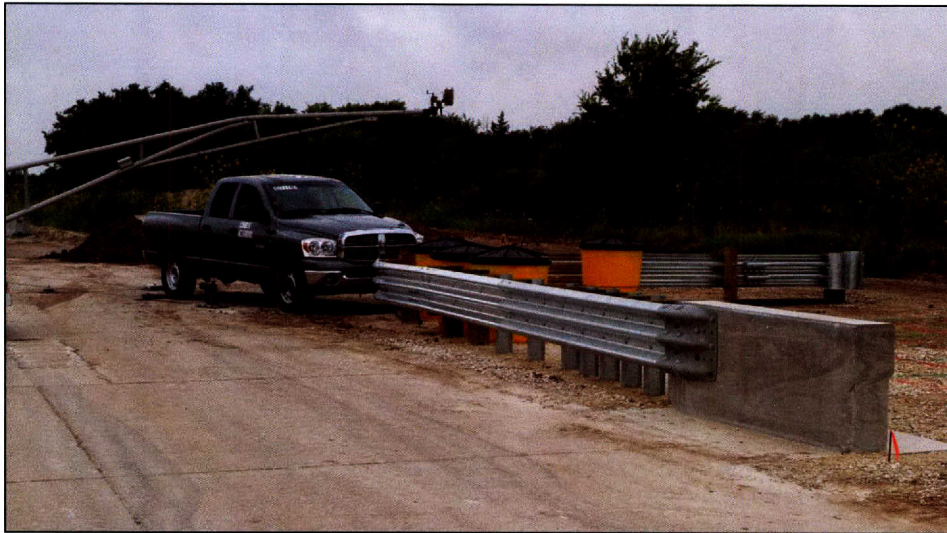
Figure 3. Short Radius Guardrail System.
