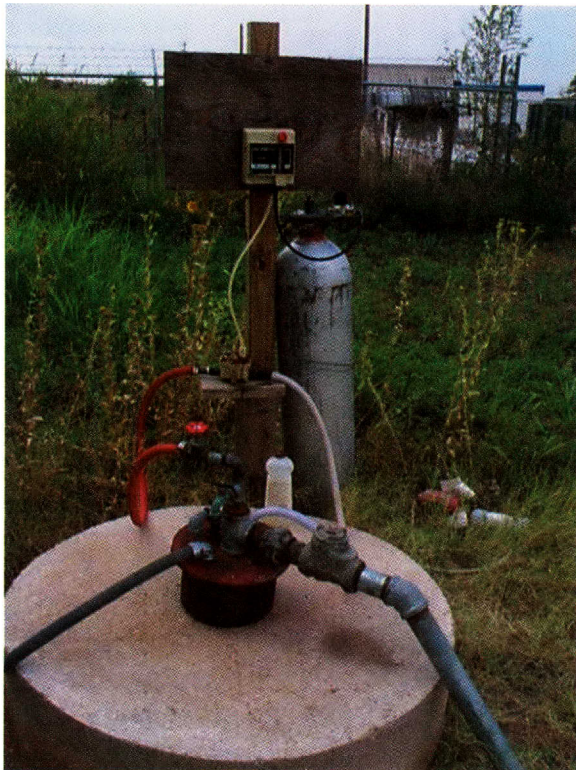
Figure 5. Do you recognize safety hazards in this photograph?
