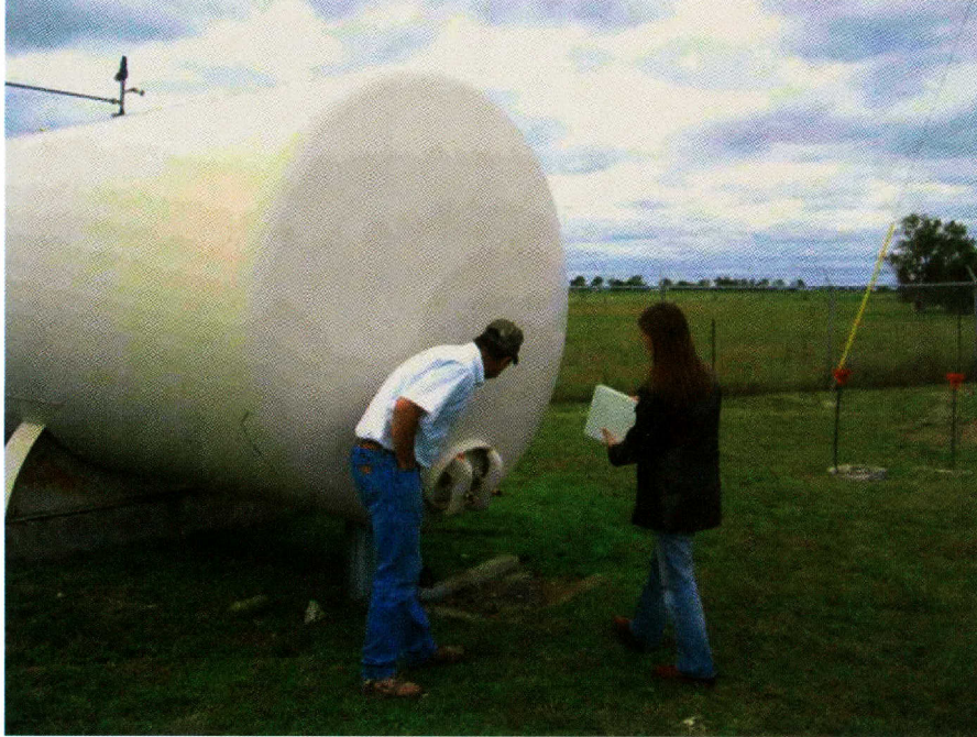
Figure 4. Checking storage and pressure tanks is an important part of every investigation.
