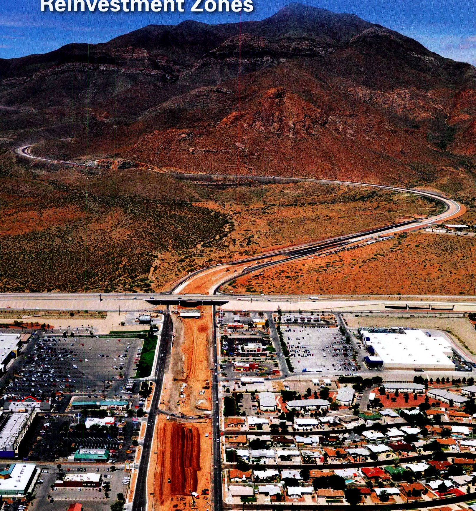
The funding generated from a transportation reinvestment zone helped build the retaining walls on the El Paso Transmountain Project.
