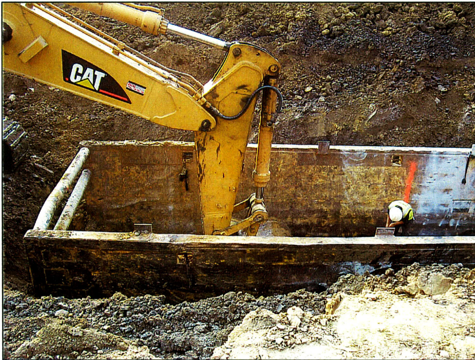
Figure 3. Metal trench box used during excavation of pipeline route. View is to the east.
