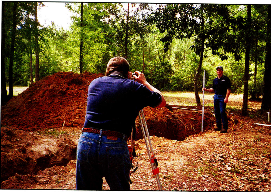
A LASER LEVEL is used to ensure the excavation is level before installing tanks.
