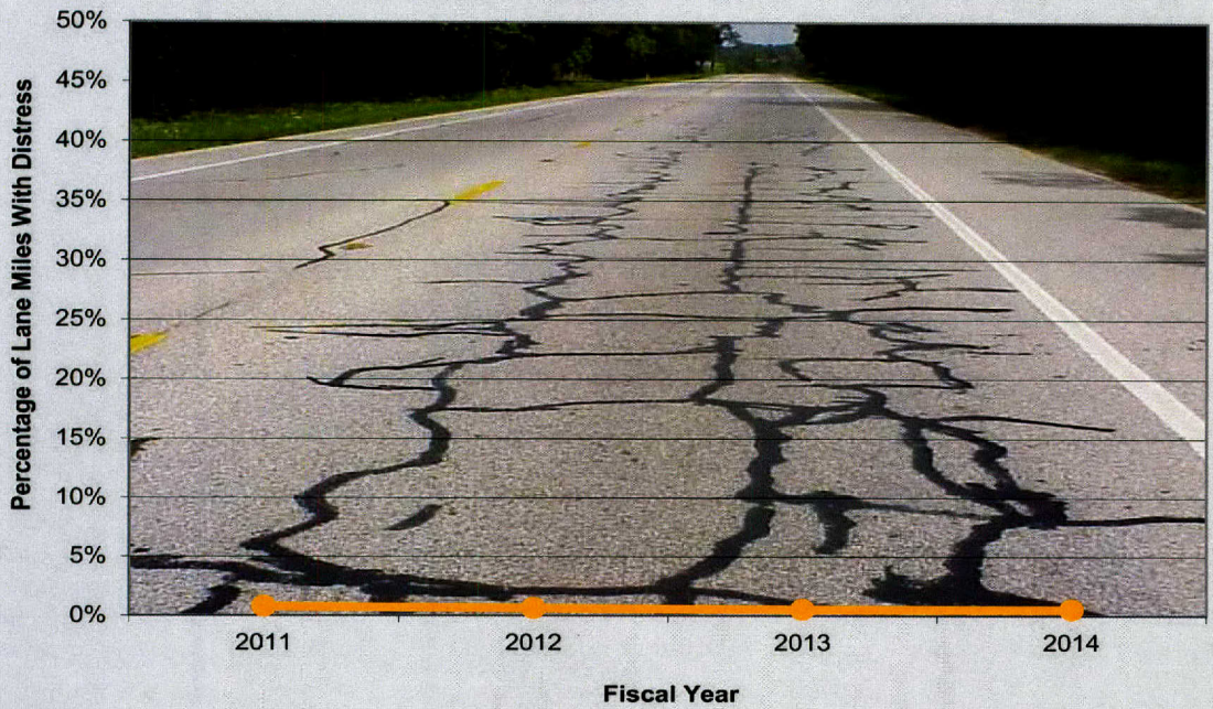
ACP Block Cracking (rated), FY 2011–2014
