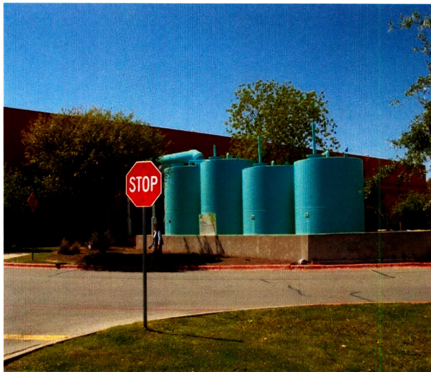
Figure 11: 28,000-Gallon Cisterns for Rainwater Harvesting on Brodie Lane, Austin, Texas
