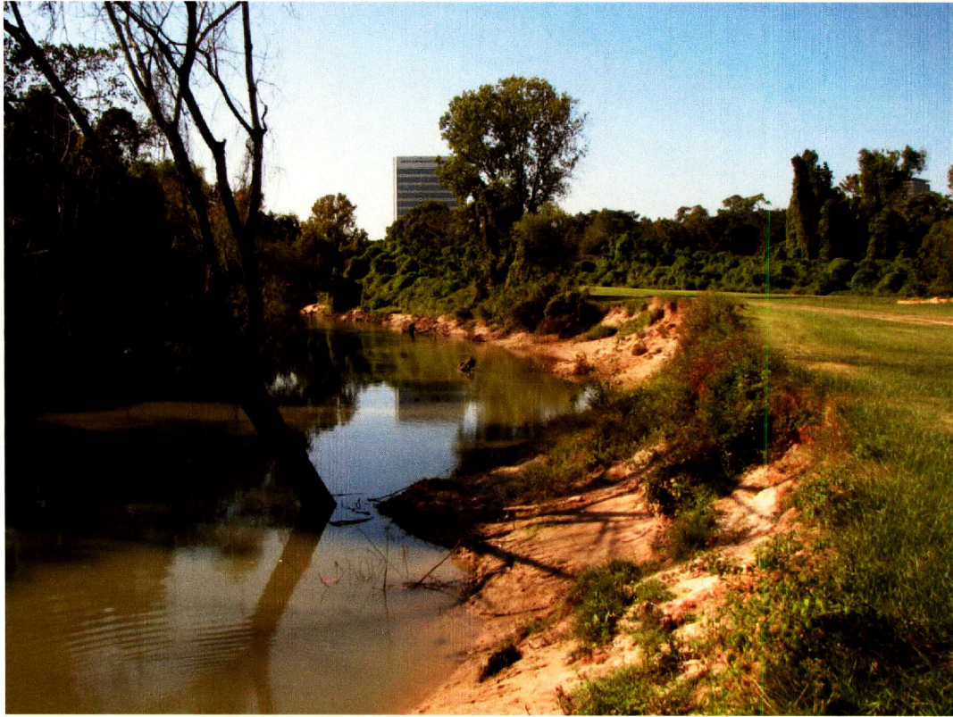
Figure B7: Bank Erosion on Buffalo Bayou at Sabine Street
