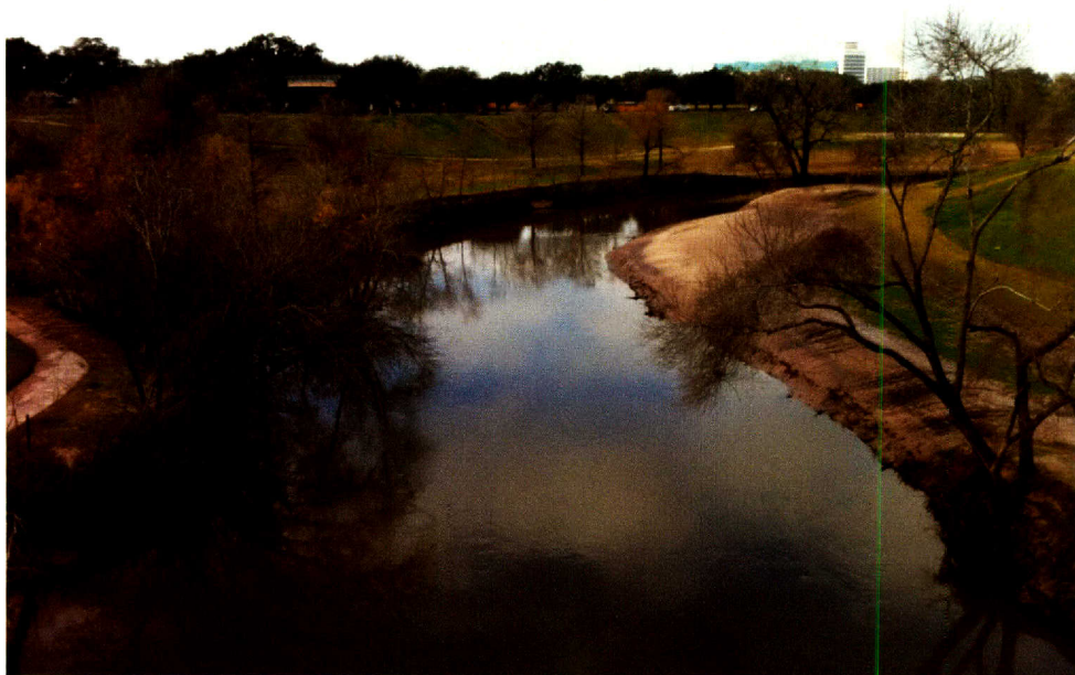
Figure B8: Buffalo Bayou at Sabine Street – Just After Construction, Prior to Planting
