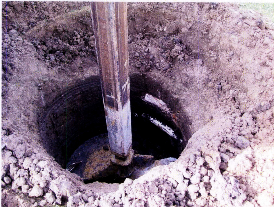
Figure 7. Structure 2/4 foundation hole showing buried West Fork soil (PVC pipe may be seen in the right side of the foundation hole), facing northwest.
