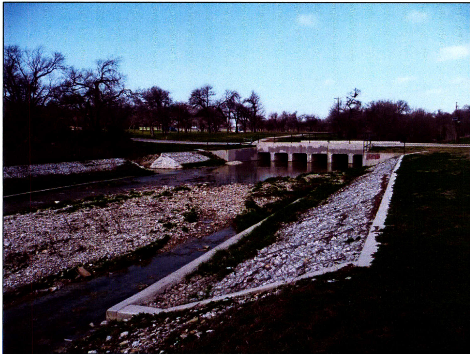
Figure 7. Overview of area south of Macie Avenue Bridge showing typical erosion control measures along Marine Creek, facing north.
