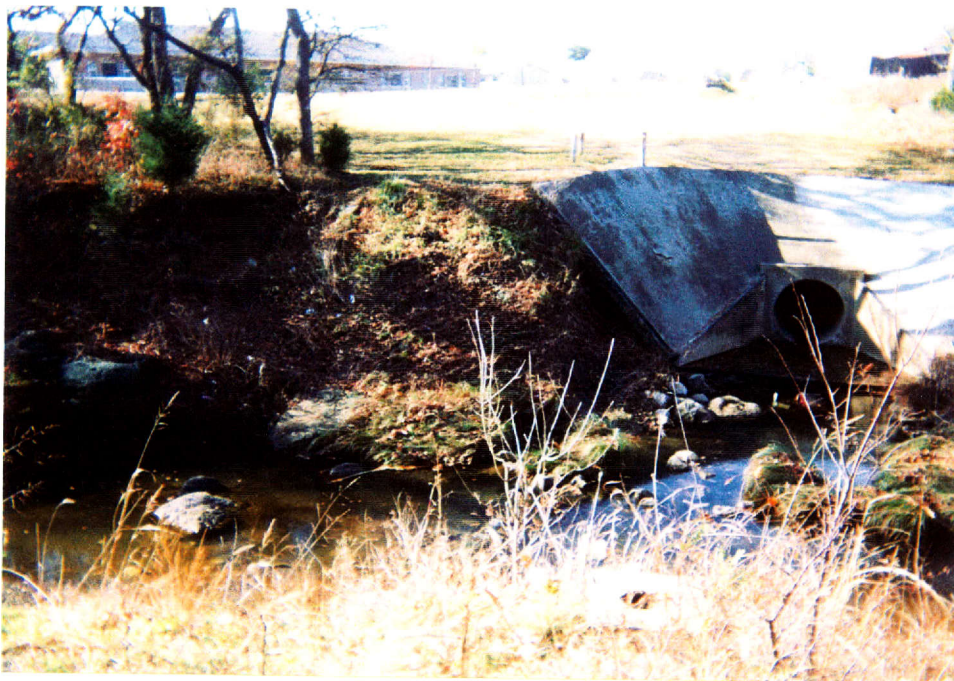
Figure 3. Above ground gas pipeline and concrete erosion guard on the southwest bank of Timber Creek. Shovel test 8 was placed between the concrete guard and trees. View is to the southwest.
