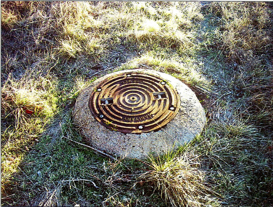
Figure 5. Manhole from sewer pipeline paralleling the north bank of Trail Creek. View is to the east.
