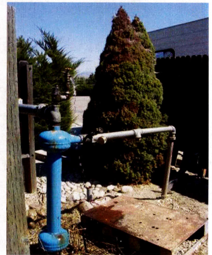
Figure: The wellhead on your property will typically include a pipe leading to your pressure tank.
