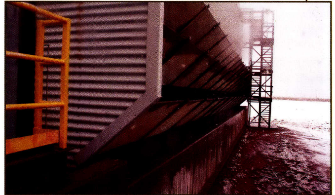
Figure 11. Water cooling tower at the Levelland Hockley County Ethanol plant.
