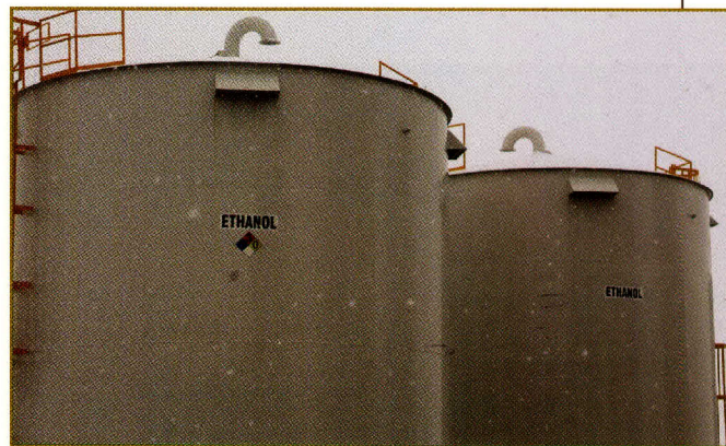
Figure 6. Ethanol storage tanks at the Levelland Hockley County Ethanol plant.
